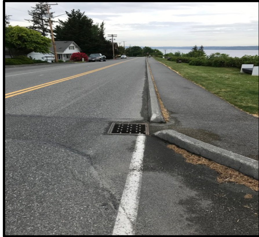
Walkway on 6 th Street and South side of Edgecliff w/o walkway
