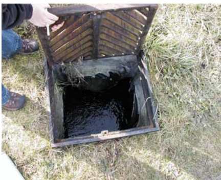
City of Langley stormwater catch basin
